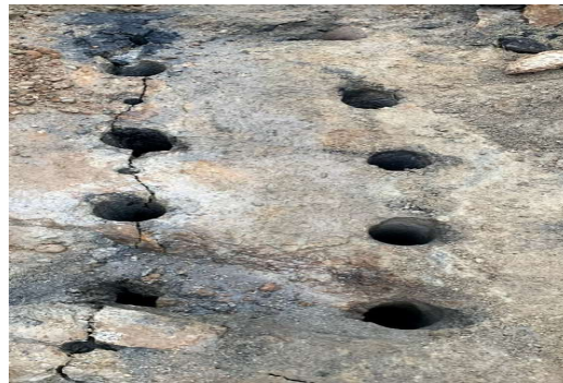
Figure 10: Post blast: Crack generated through Modified presplit Blast.
