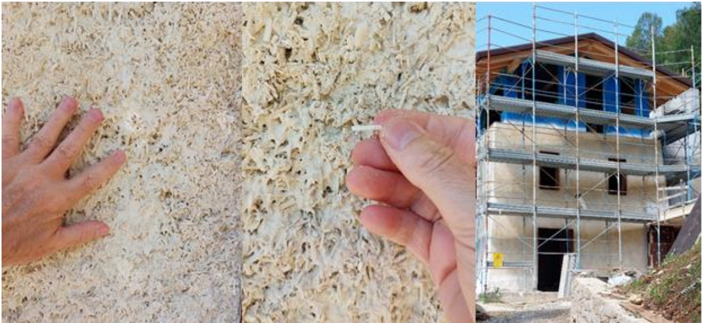
Figure 8: Showing hempcrete spray applied to existing masonry wall in rural house renovation. Senini-Tecno Canapa northern Italy [Source Author].
