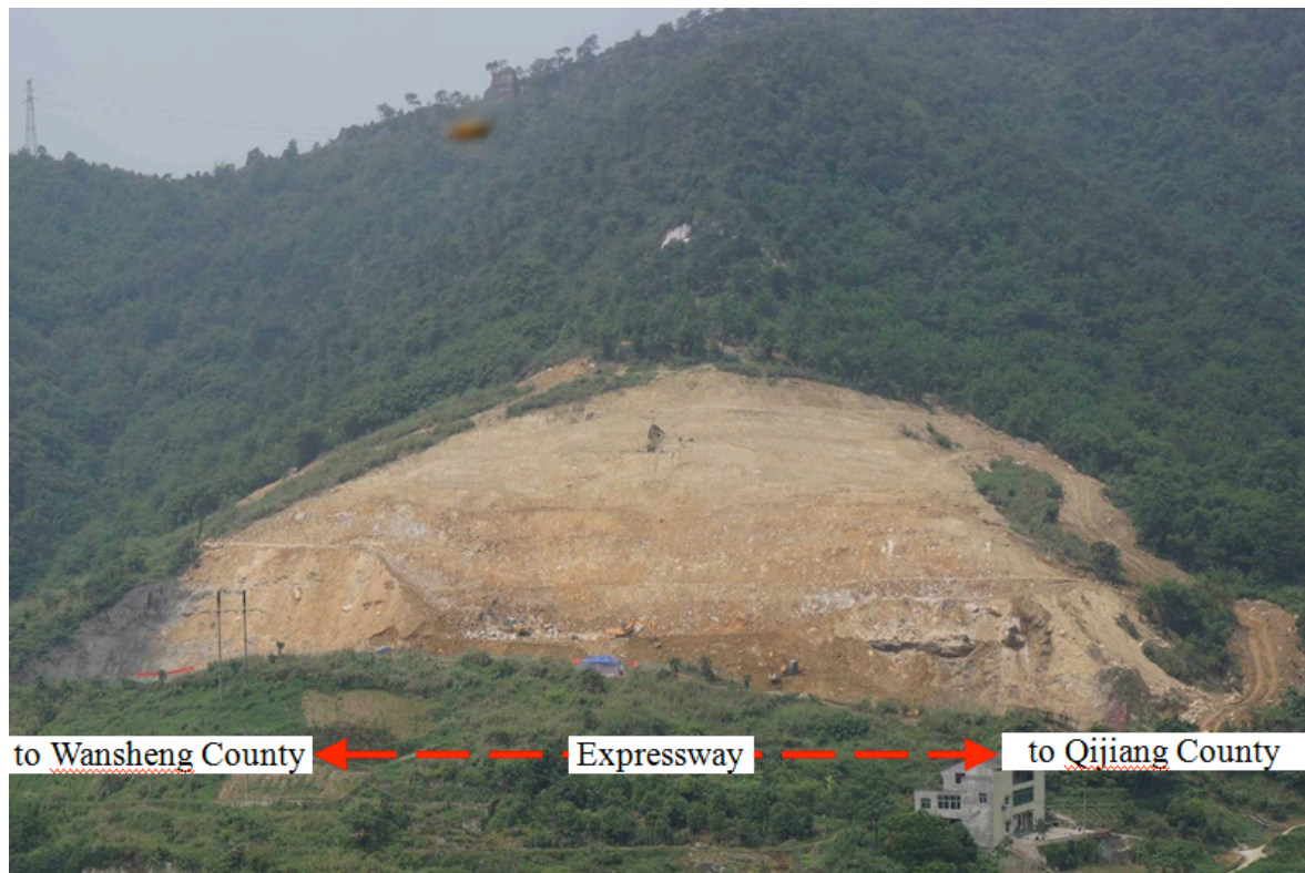
Figure 4: Photo of landslide after excavating superficial unstable materials.
