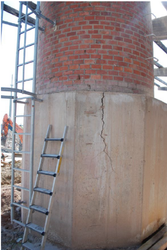
Figure 3: Cracks in the chimney.
